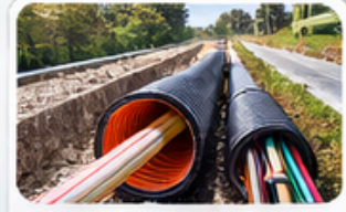
Optical Fiber Cable Network
